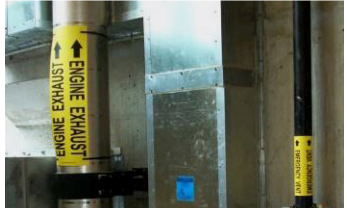
A fire-rated pipe enclosure
